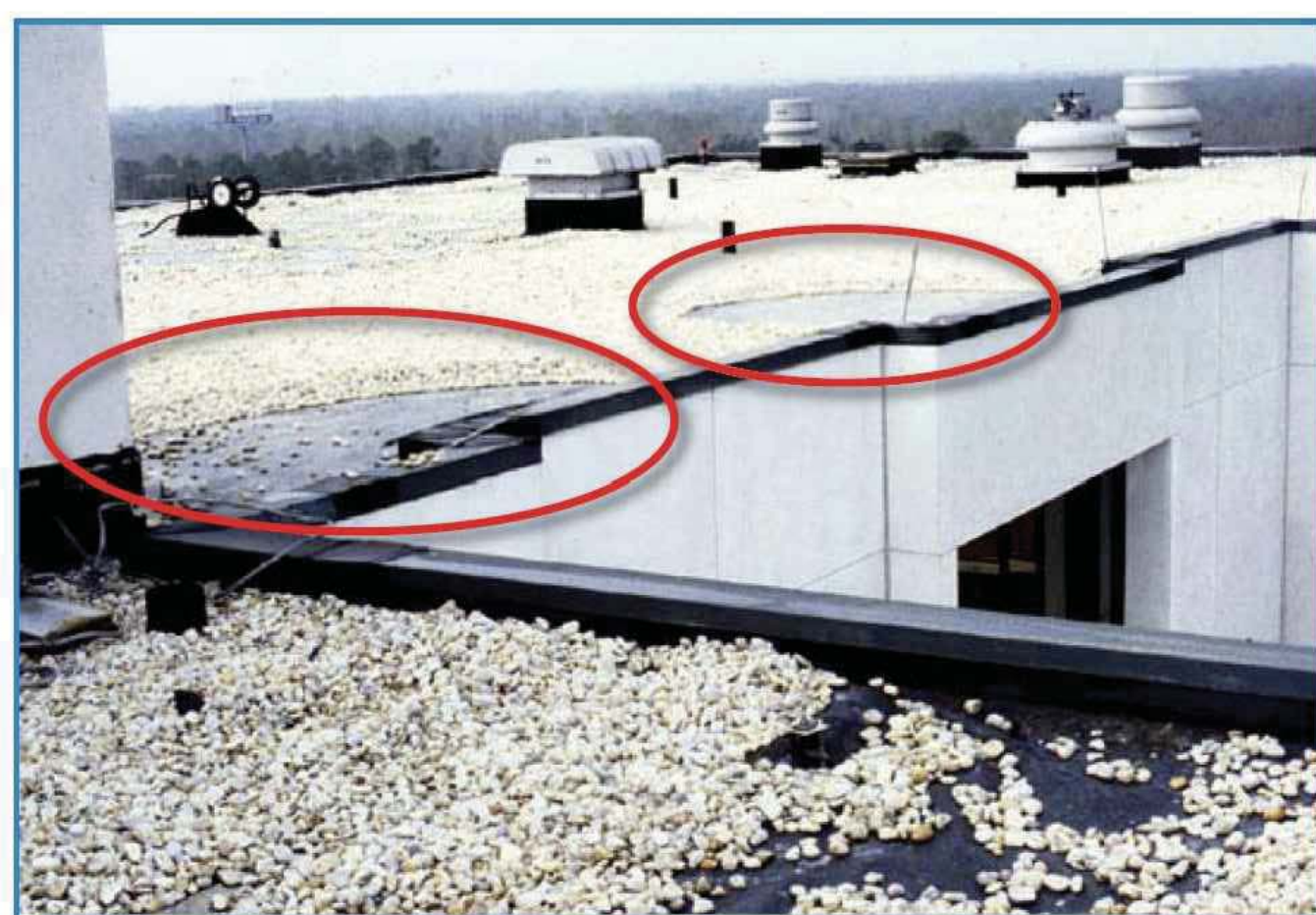
Figure 3-9: Aggregate blow-off associated with building irregularities. Hurricane Hugo (South Carolina, 1989)
