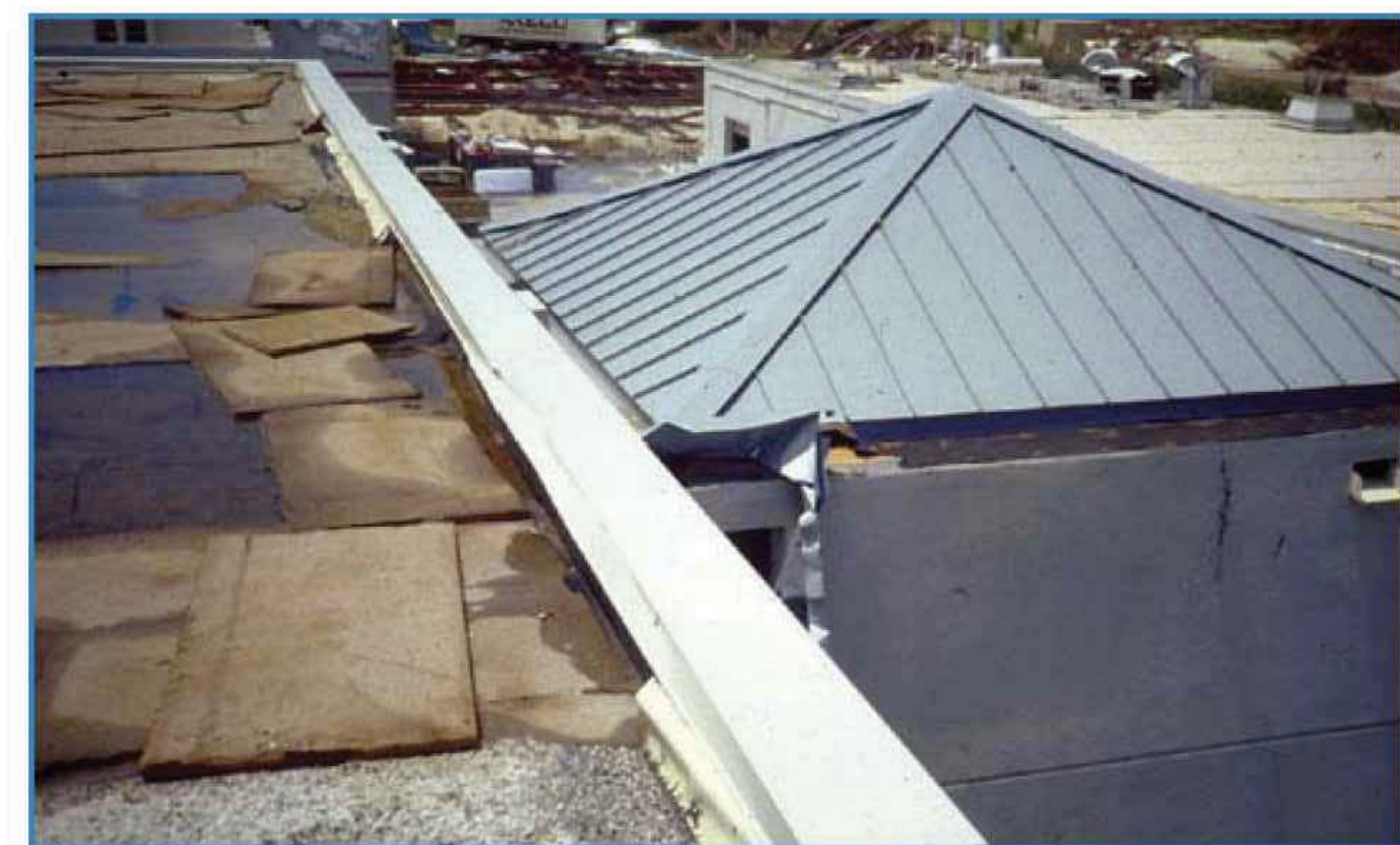
Figure 3-10: The irregularity created by the stair tower (covered with a metal roof) caused turbulence resulting in wind speed-up and roof damage. Hurricane Andrew (Florida, 1992)
